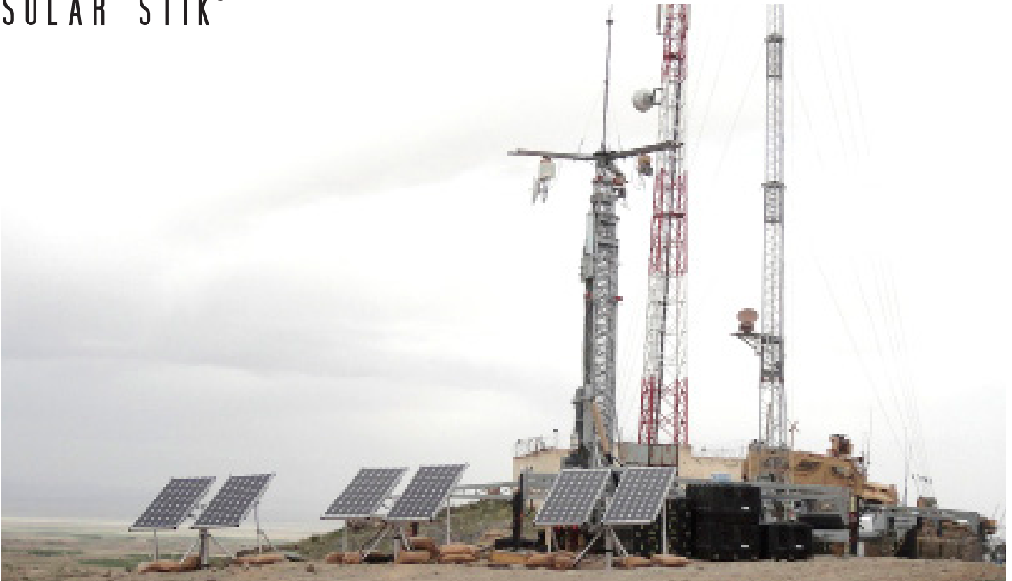
Figure 1 - The Solar Stik 3.0 kW TQG Hybrid Power System powering ISR assets
