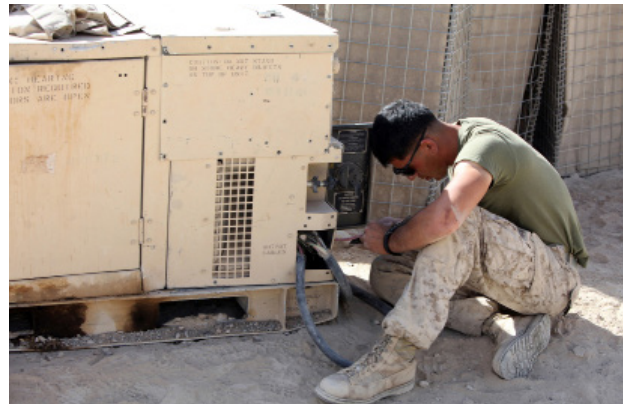
Figure 3 - Marine working on broken generator
