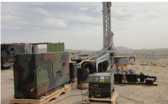
Figure 6 - The 3.0 kW TQG Hybrid Power System replacing the 60 kW Generator
