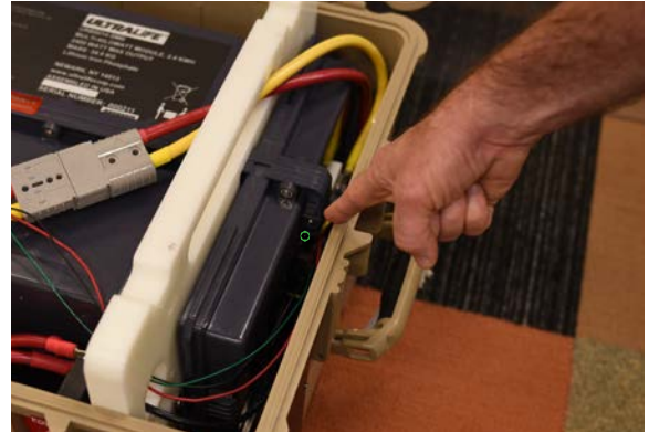
Figure 16. BMS LED indicator light
