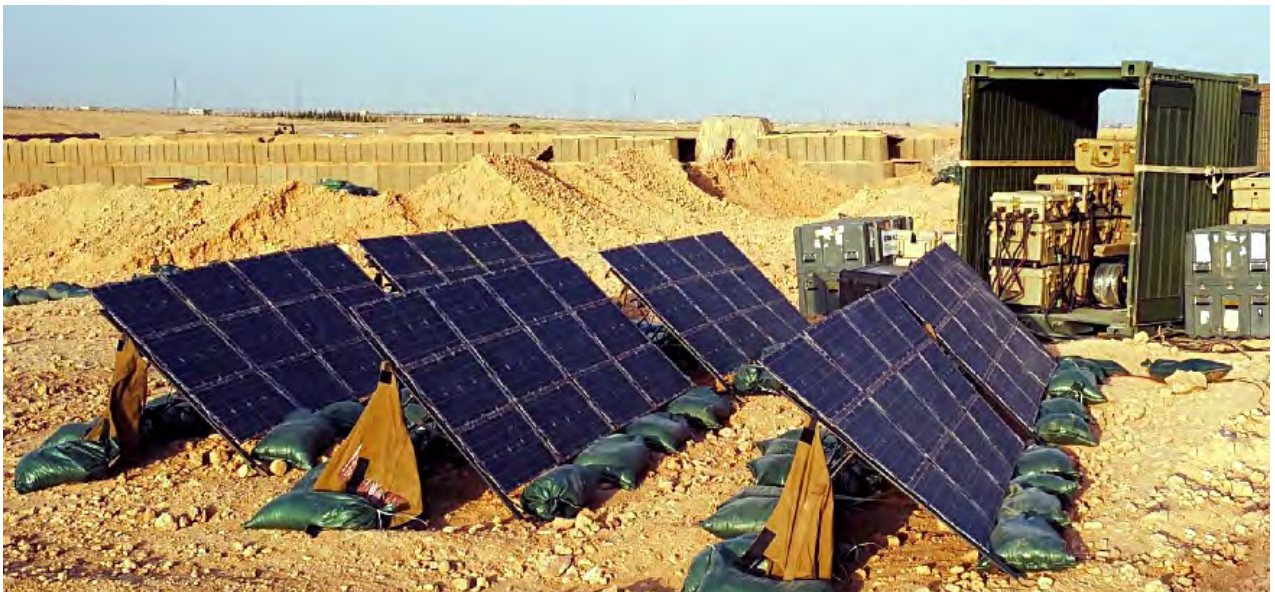
Figure 3. Hybrid Power System in Operation
