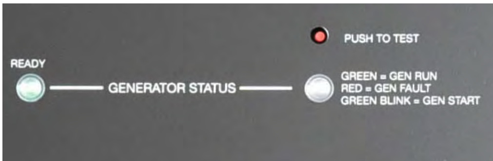
Figure 24. Generator Status LEDs
