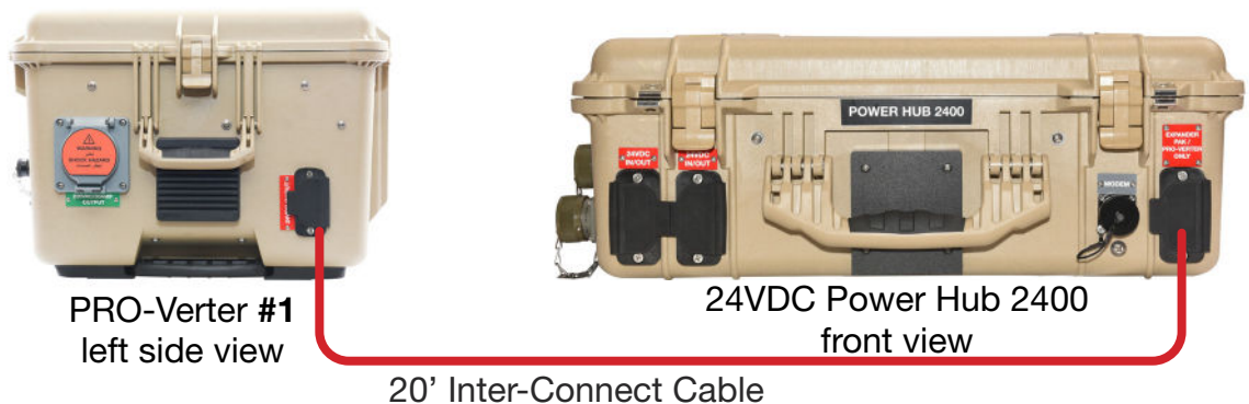
Figure 14. PRO-Verter to Power Hub connection
