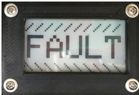
Figure 17. Battery Status Indicator - home page unattended fault warning
