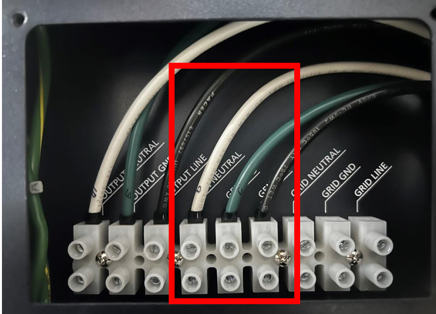
Figure 4 - magnified view of Inverter/Charger Terminal Block with incorrect wiring.
