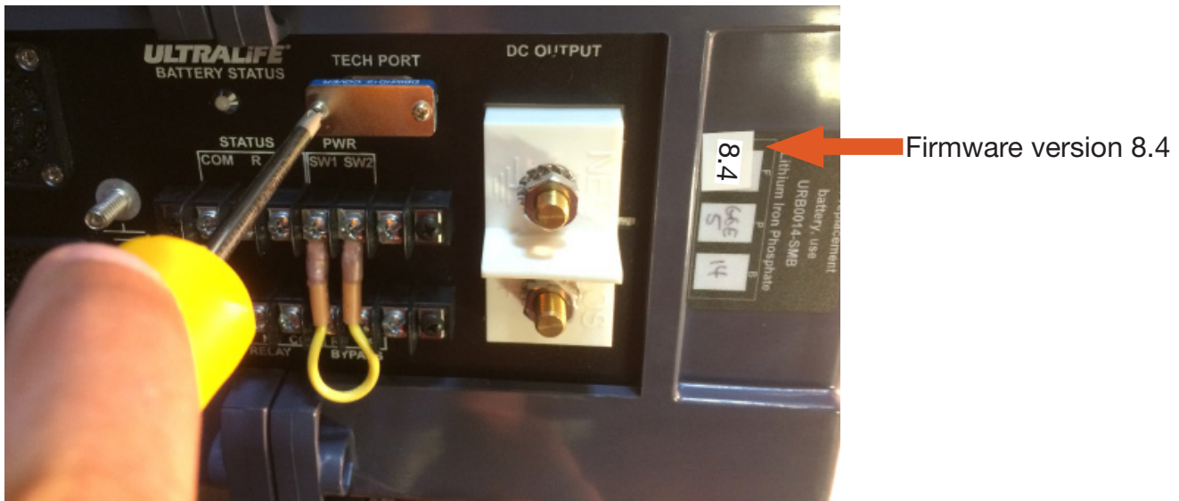
Figure 29. Removing Tech Port cover
