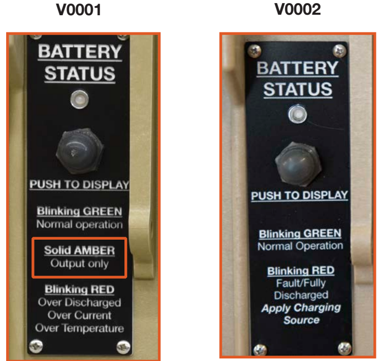
Figure 26. V0001 and V0002 Battery Status LED placards
